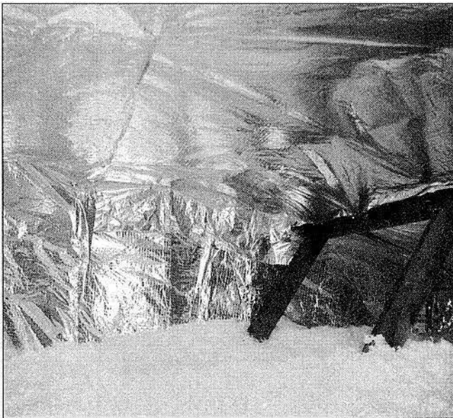
This attic would be a ham's nightmare. The proliferation of foil-backed insulation makes it useless as a location for antennas.
